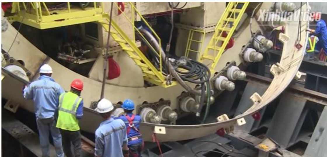
Image: Workers engaged in the construction of the Jakarta-Bandung High Speed Railway, a major BRI project in Indonesia. (Source: Youtube / Xinhua )
