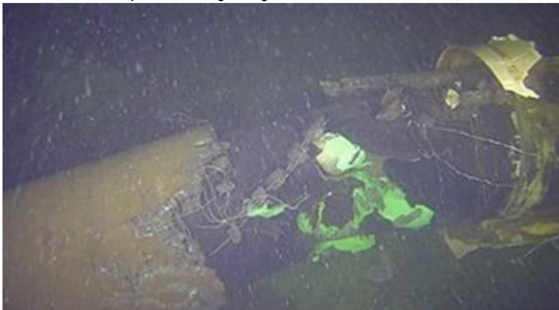
Figure 2: Balticconnector Pipeline Following Damage From Chinese Merchant Vessel, October 7, 2023
